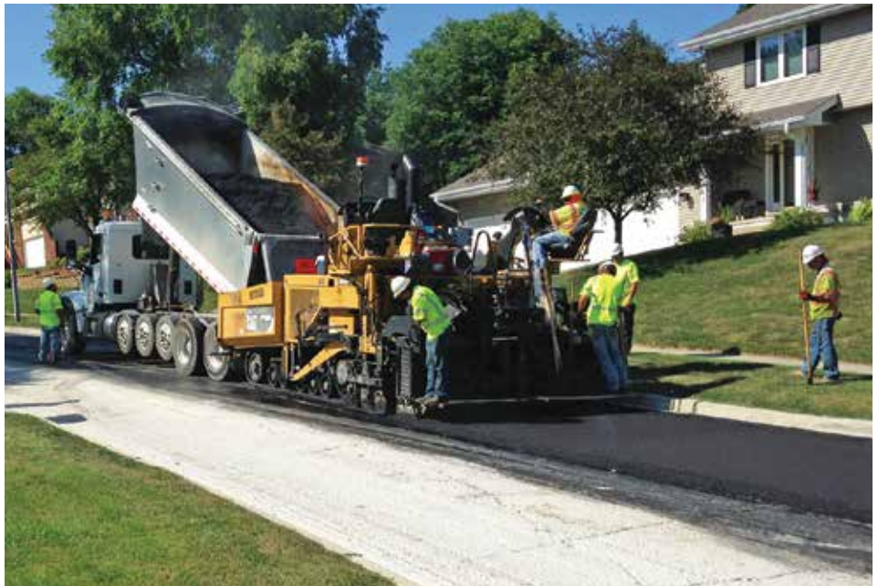
Des Moines Asphalt and Paving placing the Asphalt Interlayer for the City of Clive.
