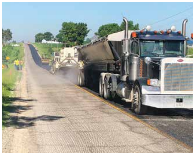
Hamilton County HIPRO project constructed by Mathy Construction Co. in June of 2018.
