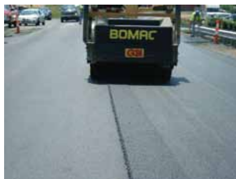
Vibratory compactor passes over an 18-inch-wide section of uncompact material along the joint. Note that the roller pass lips over the cold mat.
