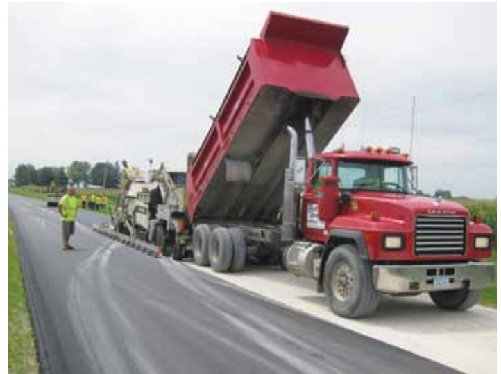
A Fort Dodge Asphalt paving crew paves over the rock interlayer on Webster Co. road P59 on the same day.
