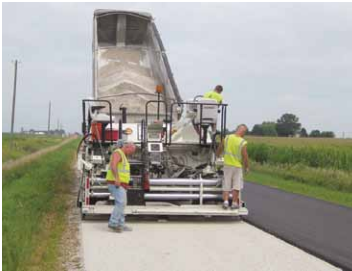
A Fort Dodge Asphalt crew places a rock interlayer on Webster Co. road P59 in 2010.
