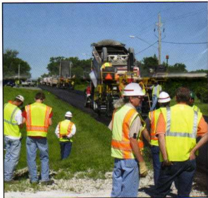
Members of Polk Co. and the IDOT watching the placement of WMA by Des Moines Asphalt.
