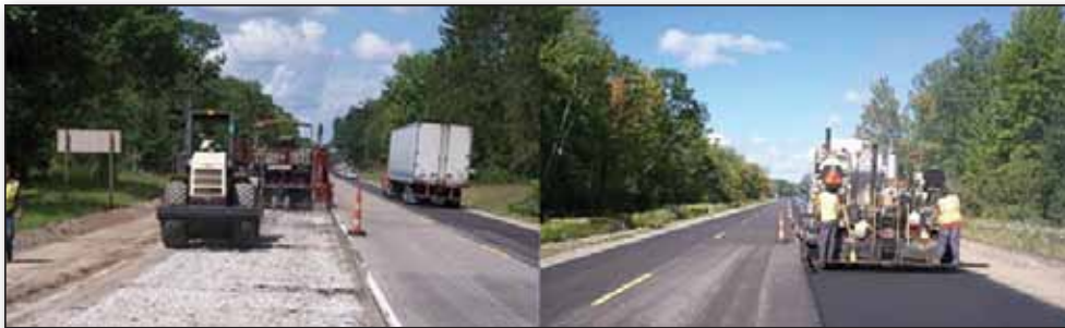
Rubblization allows lanes of traffic to remain open during pavement reconstruction. (Images courtesy of FHWA)
